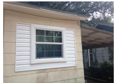
EXAMPLE OF A LOW-INCOME QUALIFIED HOME REPAIR IN THE STATE HOUSING INITIATIVE PARTNERSHIP (SHIP) PROGRAM. PHOTO CREDIT: STAFF
