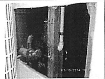
Area of leak on left, close up of leak above. Opening in drywall as result of repair earlier in the day.
